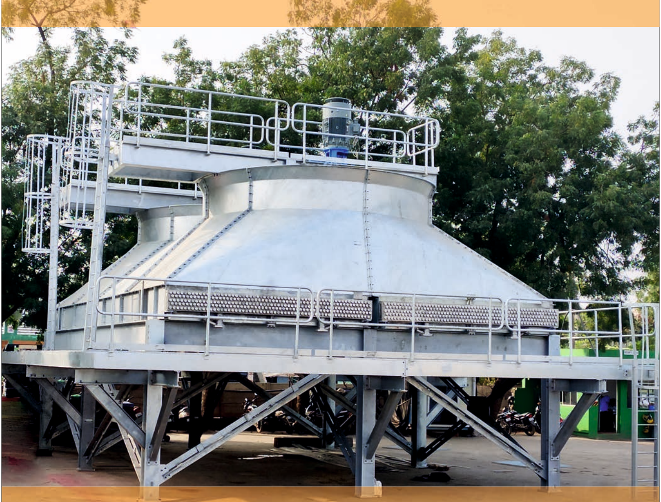
Air Cooled Heat Exchanger
