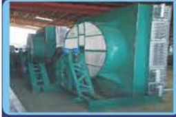
CNG Air Exchangers
